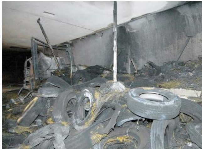
Fig. 3. Fire accident in the Fréjus Tunnel (France) on 4.6.2005
