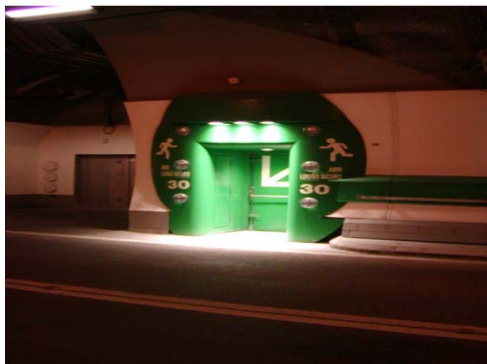
Fig. 5. Upgrading of tunnels: Well marked emergency exit in the re-opened Mont Blanc Tunnel (France/Italy)
