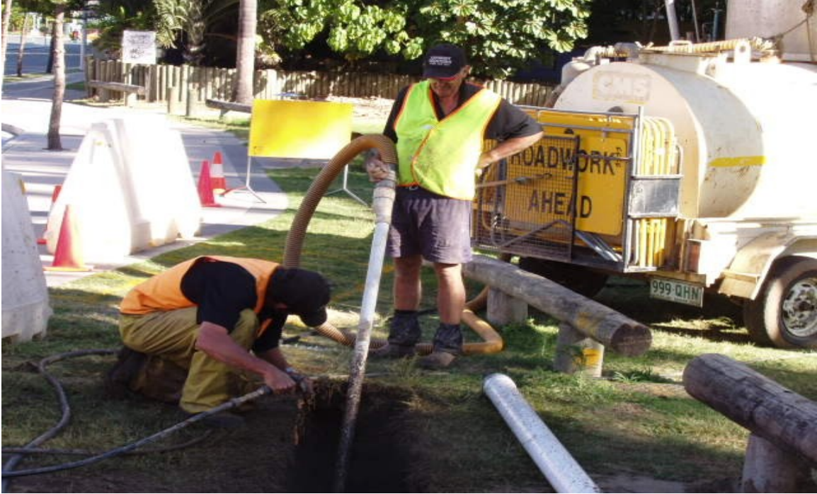
The Photograph Shows the Compact System Using Water Jetting With Vacuum Suction. Note the small tank in the background.
