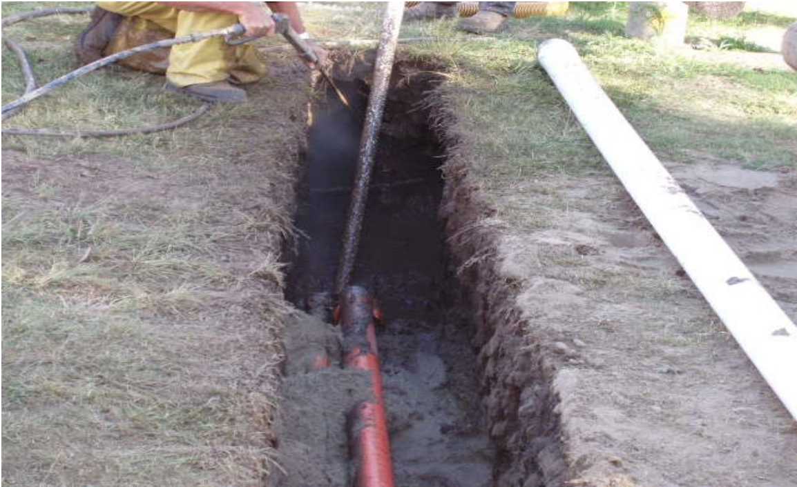
The Photograph Shows the Exposed Service Duct. Notice the Neat and Clean Surrounding.
